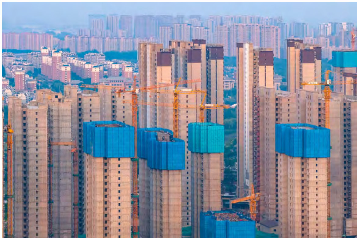
A real estate complex under construction in Huai'an, Jiangsu province. The property sector, a growth engine for the economy, is suffering from long-term oversupply © Costfoto/NurPhoto/Getty Images
