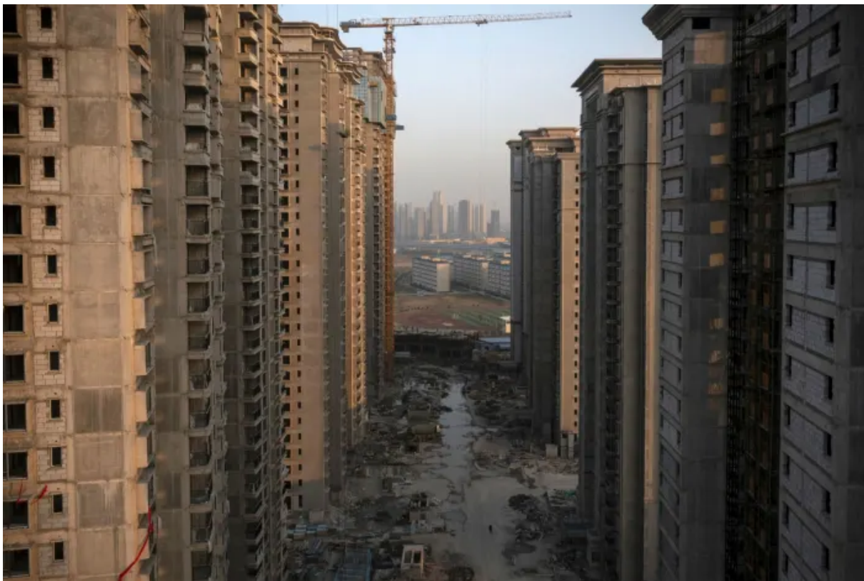
Unfinished apartment buildings at the construction site of an Evergrande development in Wuhan, China © Andrea Verdelli/Bloomberg
